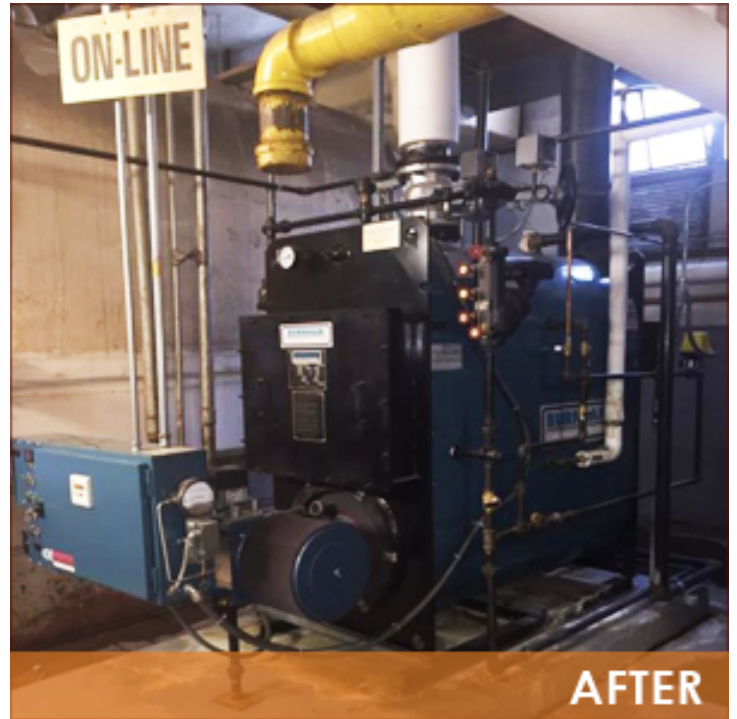
Burnham steam boilers and Webster ultra low NOx burners save energy and reduce pollutants
