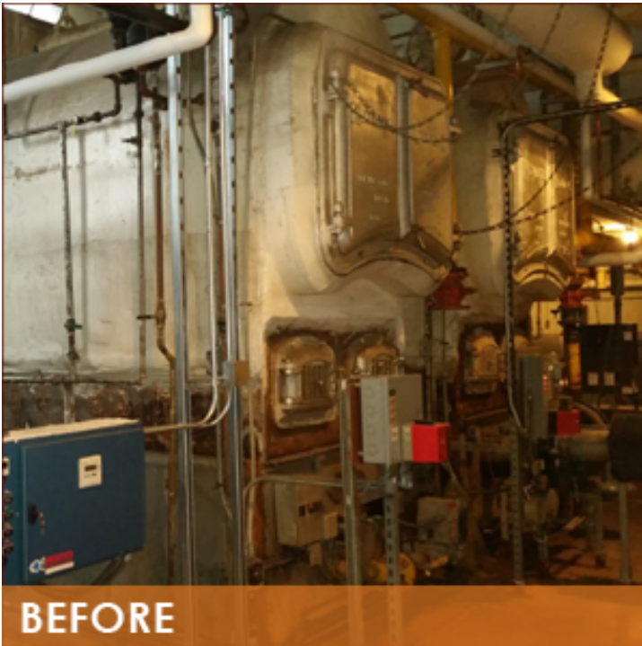
70-year-old Kewanee boilers urgently needed replacement.
